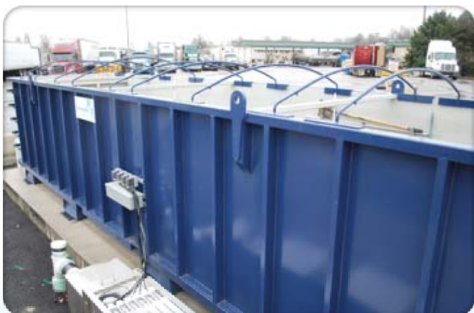
StormwaterRx Aquip system near truck parking lot and fuel island
